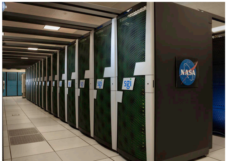
The Pleiades supercomputer at the NASA Advanced Supercomputing (NAS) Facility includes racks based on Intel's latest Westmere processor. During 2010, a series of expansions brought Pleiades to 10,816 nodes (101,120 cores). Photo by Dominic Hart, NASA Ames Research Center.
